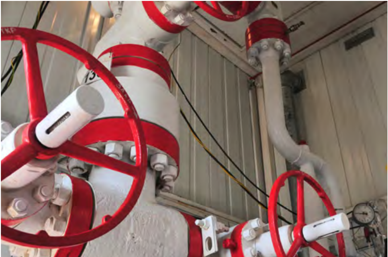
Vankor field. Well protection cover
