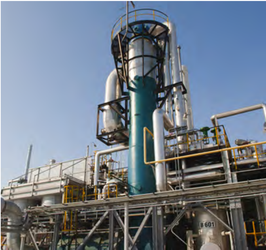
■ Samara Region. A unit for hydrogen production at the Kuibyshev Refinery
