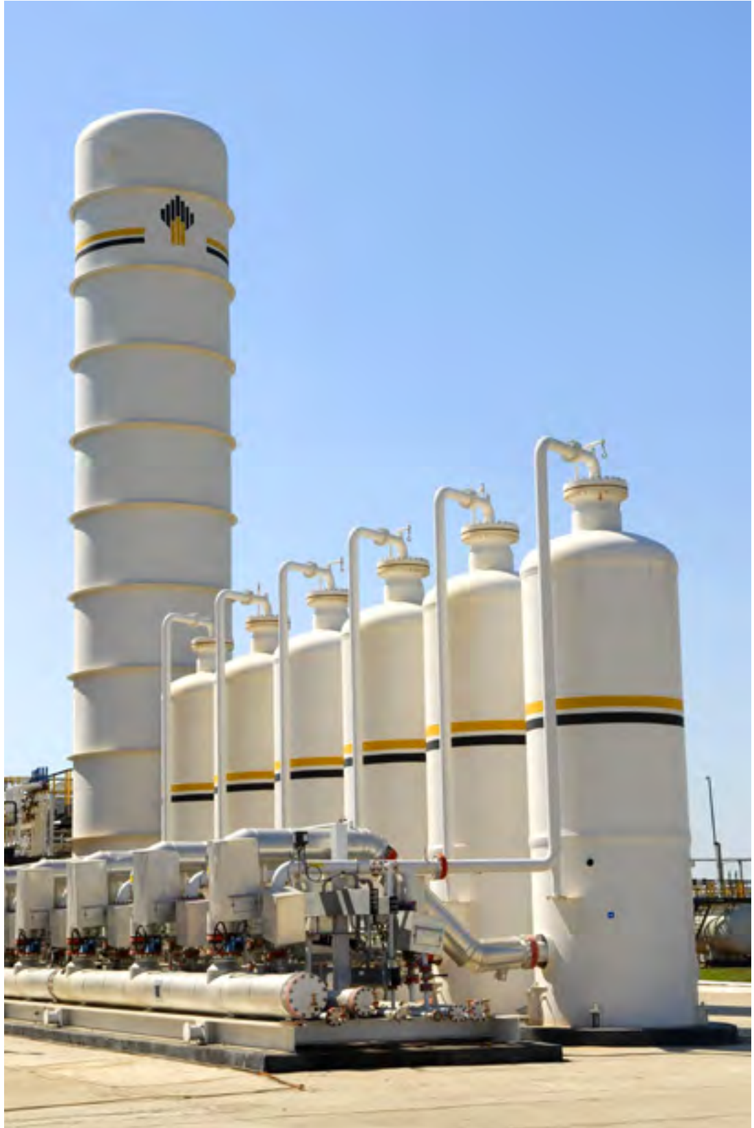
■ Novokuibyshevsk Refinery. Short-cycle adsorbion unit
